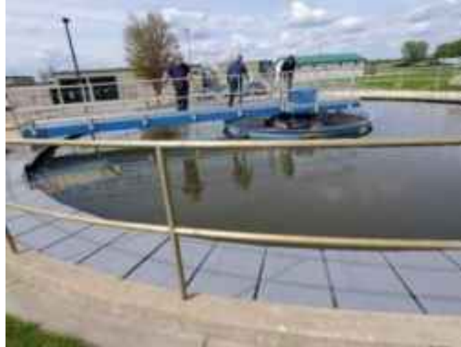
Figure 2-12: Secondary clarifier bridge and drive
