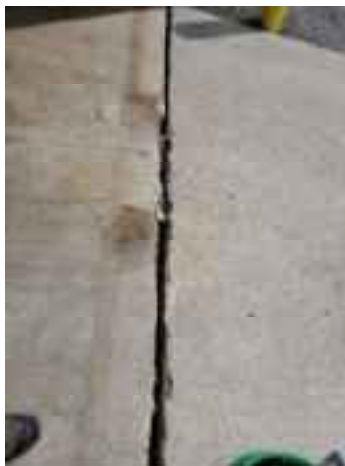
Figure 2-26: Large crack at overhead door
