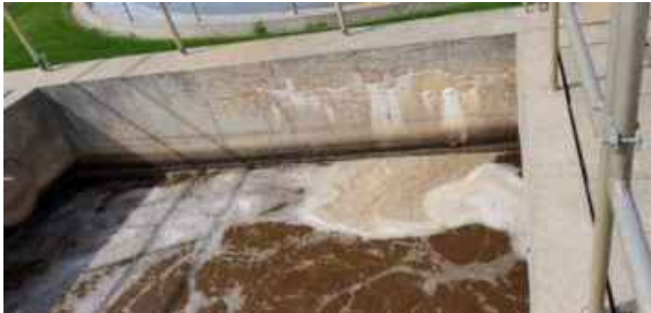
Figure 2-10: Concrete cracks in aeration tank
