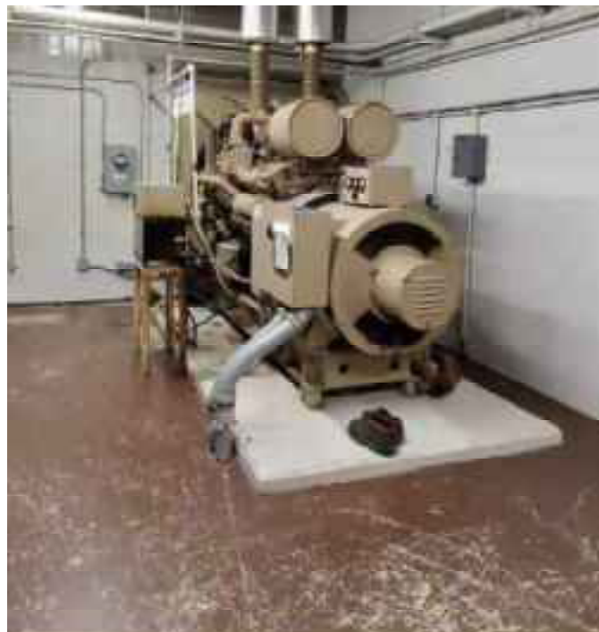
Figure 2-24: Worn painted floor in generator room
