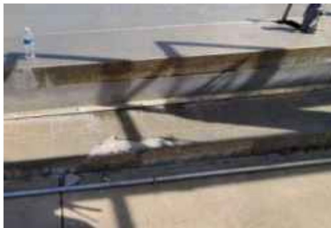
Figure 2-15: Failed concrete at south end of digesters
