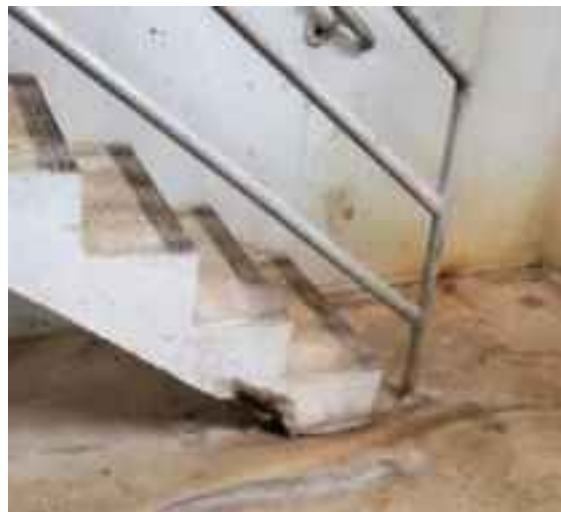
Figure 2-22: Damage to concrete stairs in influent pump station building
