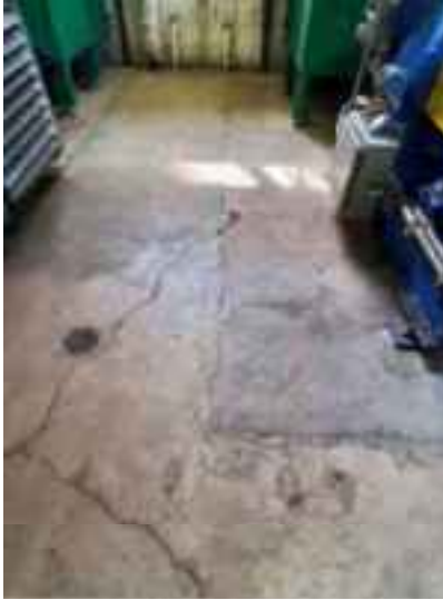
Figure 2-25: Cracks in blower room floor
