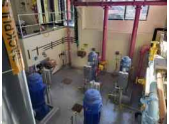
Service Water and Backpulse pumps
