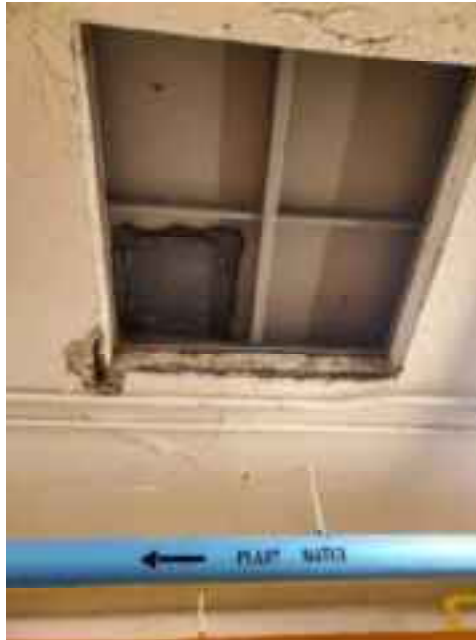
Figure 2-23: Damaged concrete around hatch
