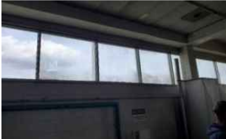
Figure 2-27: Leaking windows in centrifuge room
