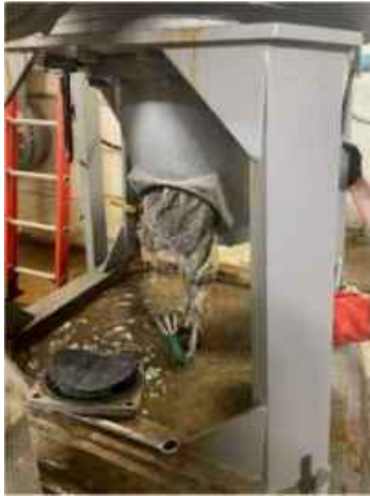
Figure 2-2: Influent pump ragging
