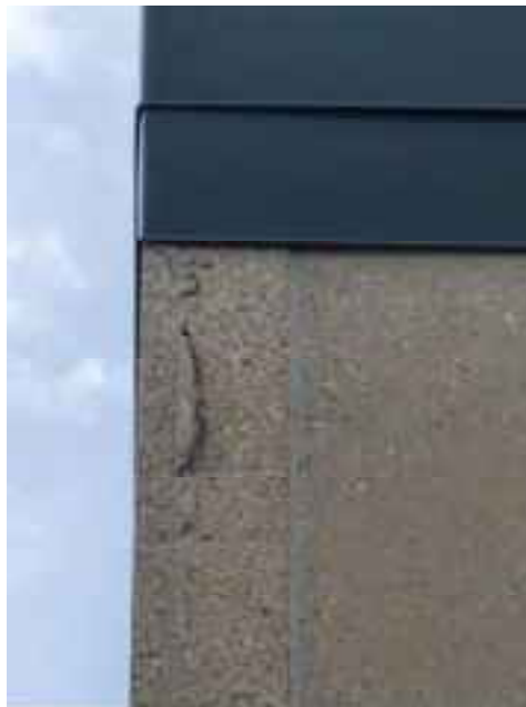
Figure 2-33: Precast wall panel cracks
