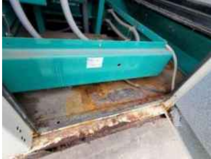
Figure 2-32: Corroded generator base
